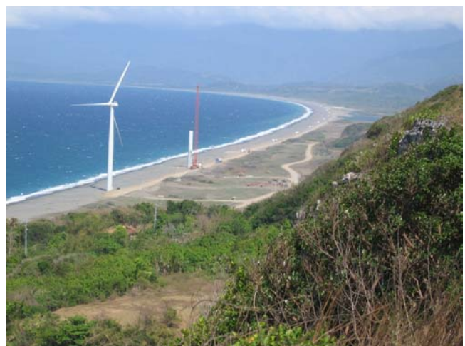
Figure 2. 25 MW Northwind Project Under Construction (March 2005). Picture copyright – Per Nørgaard, Risoe National Laboratory
