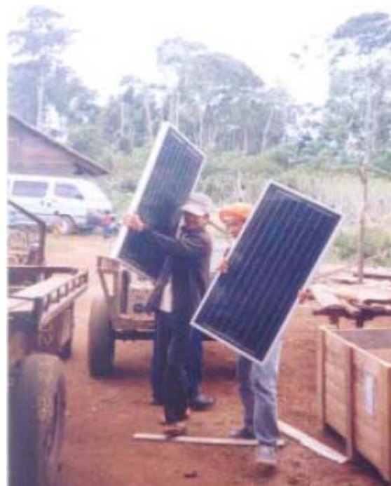
Small PV power installation in Vietnam
